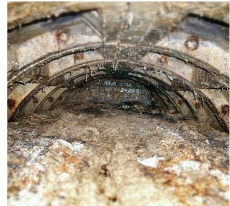
North West sewer blocked with fat
